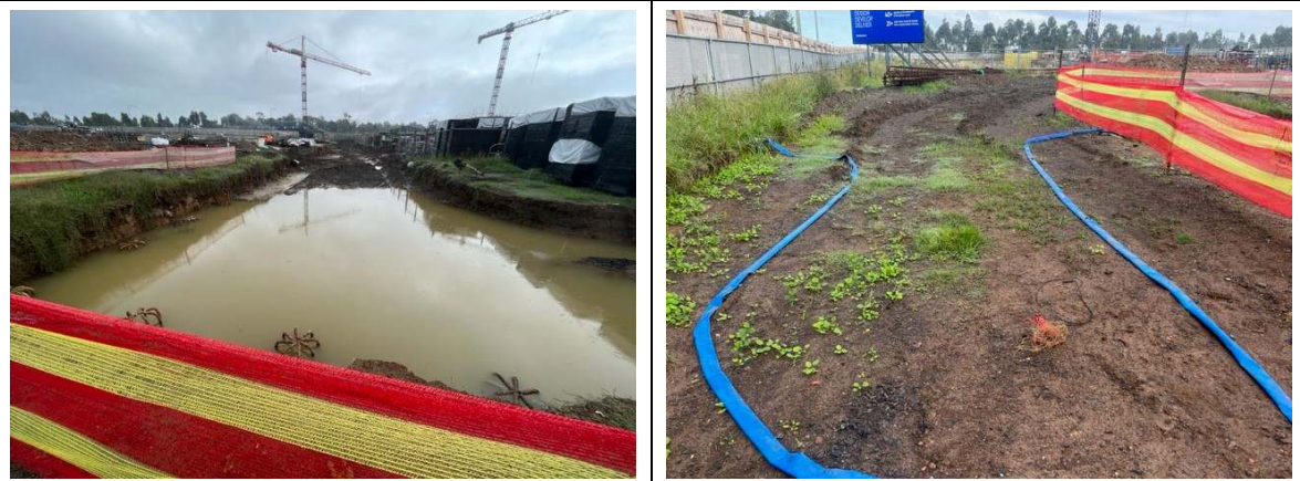
Photos 11&12: Sediment basins 1 & 2
